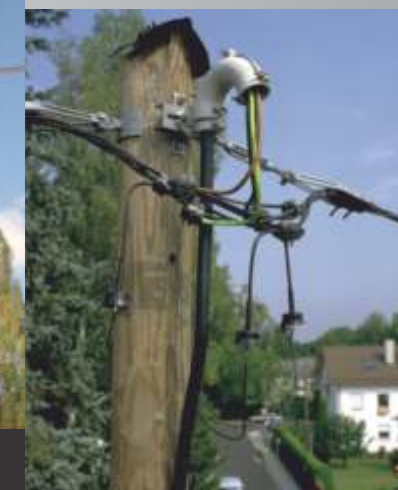
Transition : Insulated overhead lines to cables
