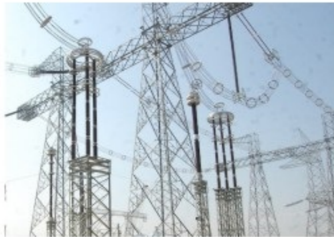
1200 kV Sub-Station at PGCIL, Bina, Madhya Pradesh
