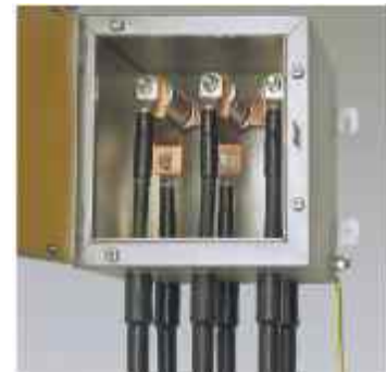
Link box installed with cross bonding cables
