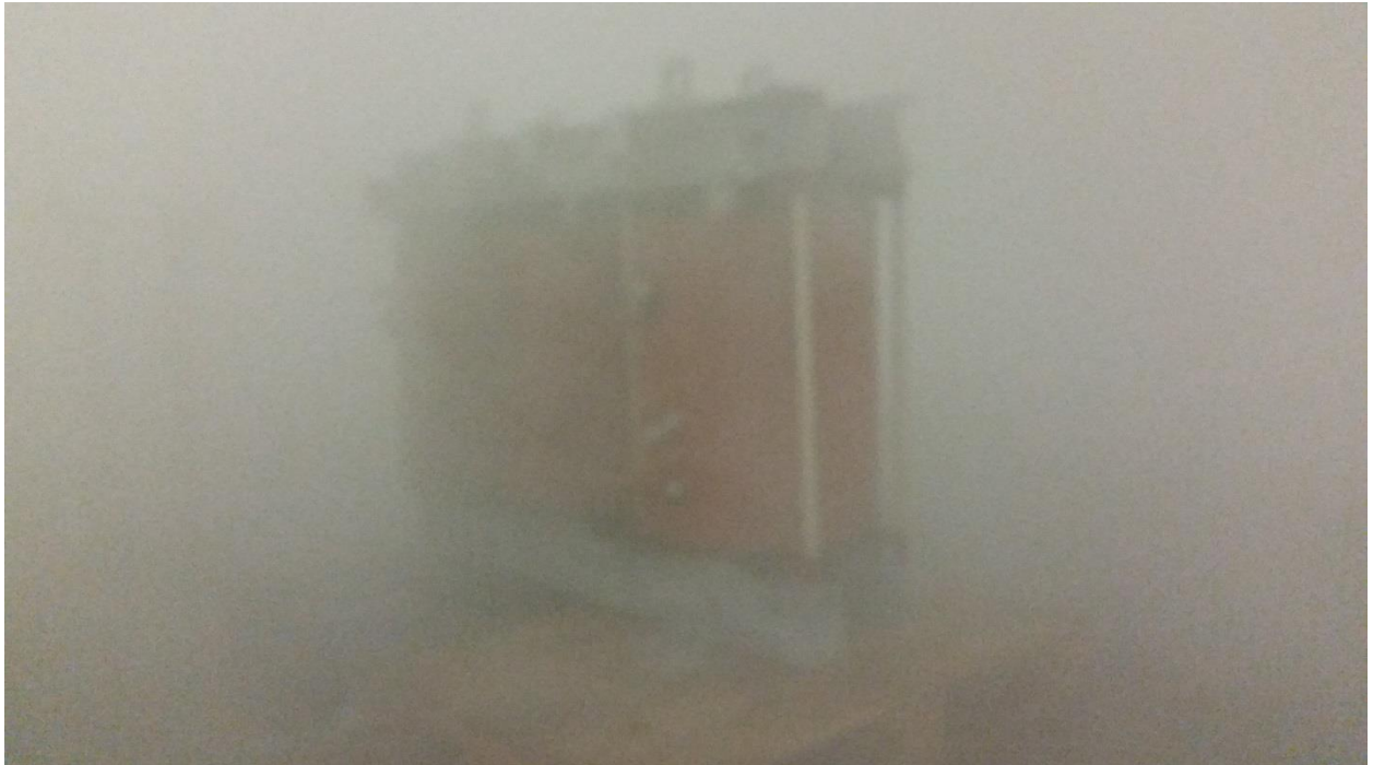
Transformer in the test bay for the condensation test.
