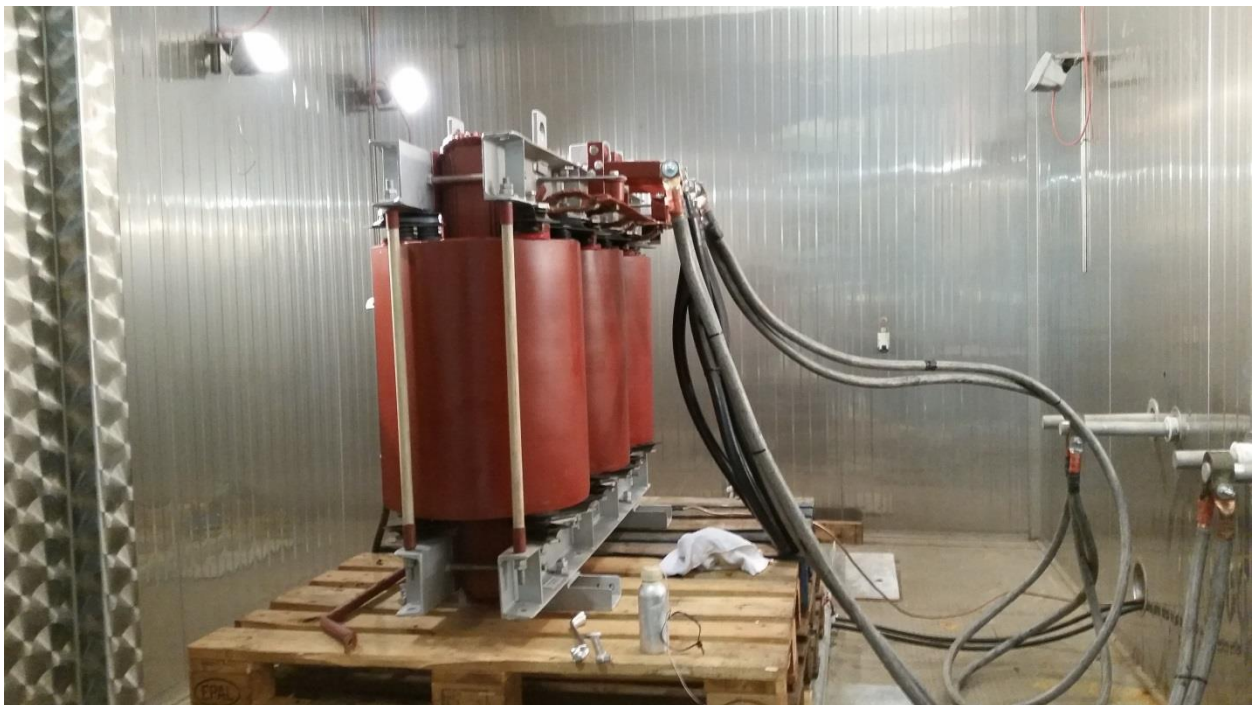
Transformer in the climatic chamber and prepared for the thermal shock test.
