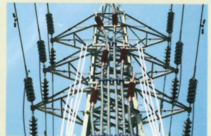
Condition assessment & maintenance of cable system
